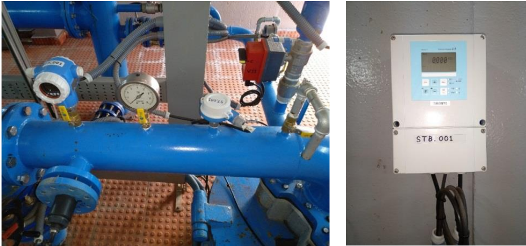
Figure 11 a) From right to left, following extraction line flow direction, sampling valve, temperature sensor, pressure gauge, manometer and turbidimeter. b) Turbidity measurement system.
