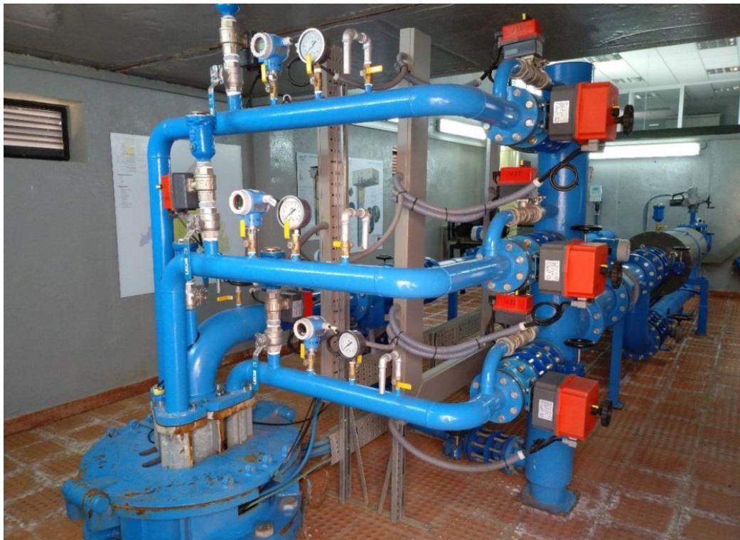
Figure 10. FE-1R recharge pipes and clamp.
