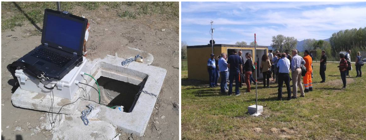
Figures 5-35 a) & b). Examples for anti-vandalism systems to protect data collection and communication elements (Serchio demo-site).
