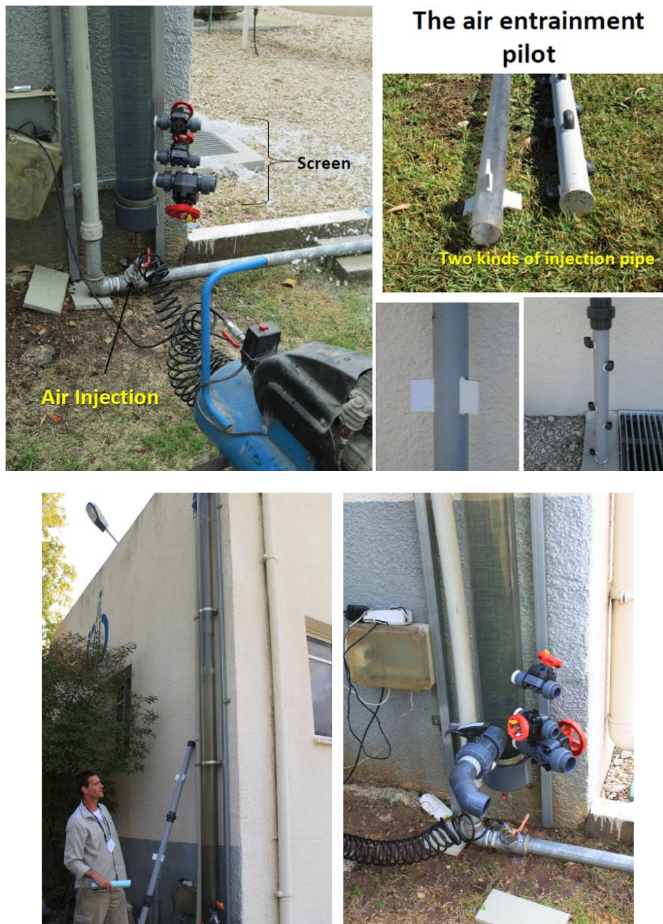
Figures 5-6 a) to c). Aspect of the air entrainment pilot to pre-treat MAR water in the heading of the circuit by means of a specific patent developed by Mekorot to reduce TOD (taken from Mekorot, 2015).
