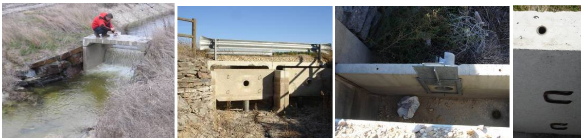
Figures 5-13 a) to d). Stopping and damming devices MAR evolution in Arenales experiences. Original design (a), The locks (gates) are raised so the water flows underneath and holes drilled halfway let water flow through the middle of the canal depth (b), the central steps are equipped with a gate to regulate the flow along the channel, that tends to occur below the contact area with the air (c). Metal screw holes practiced to remove or raise the concrete gates with a bulldozer or tractor (d).
