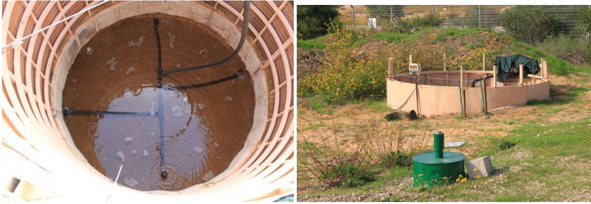
Figures 5-15 a) to c). Well design to minimize the entrance of air in the aquifer by means of a closed pipeline circuit and injection below the water table. Menashe, Israel.
