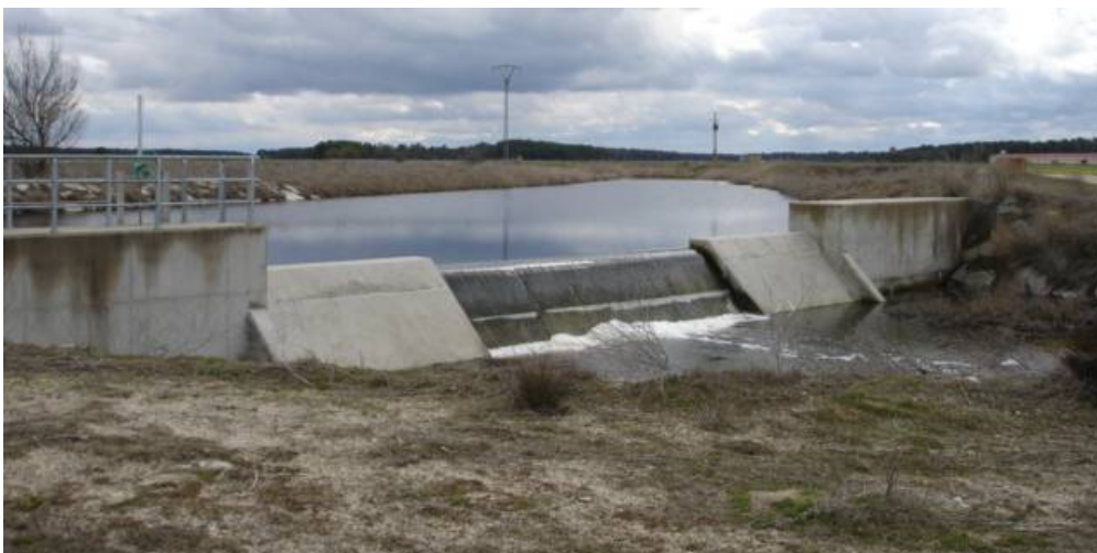
Figure 5-33. Technical solutions already deployed in Arenales Aquifer, Spain. This dam is controlling the Carracillo aquifer base level, raising the water table depth in more than 100 close wells.
