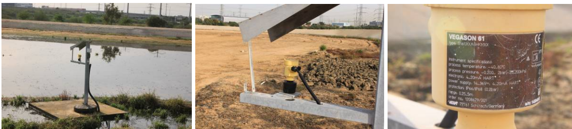
Figures 5-30 a) to c). Control of pressure devices for a MAR closed pipeline circuit.
