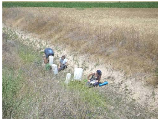
Figure 3-5. Geofabric installation in the bottom of the AR channel at Santiuste basin, Arenales demo site, in 2008.
