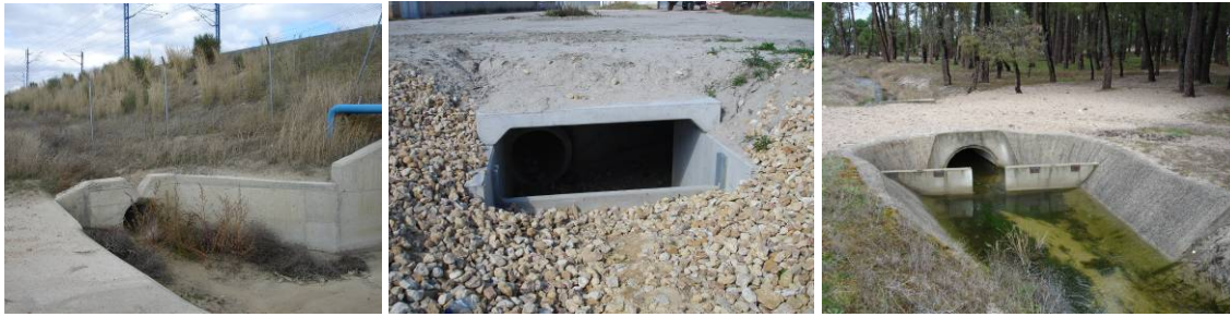
Figures 5-8 a) to c). Run-off traps, stagnation and decantation structures to pre-treat runoff water prior reaching MAR facilities
