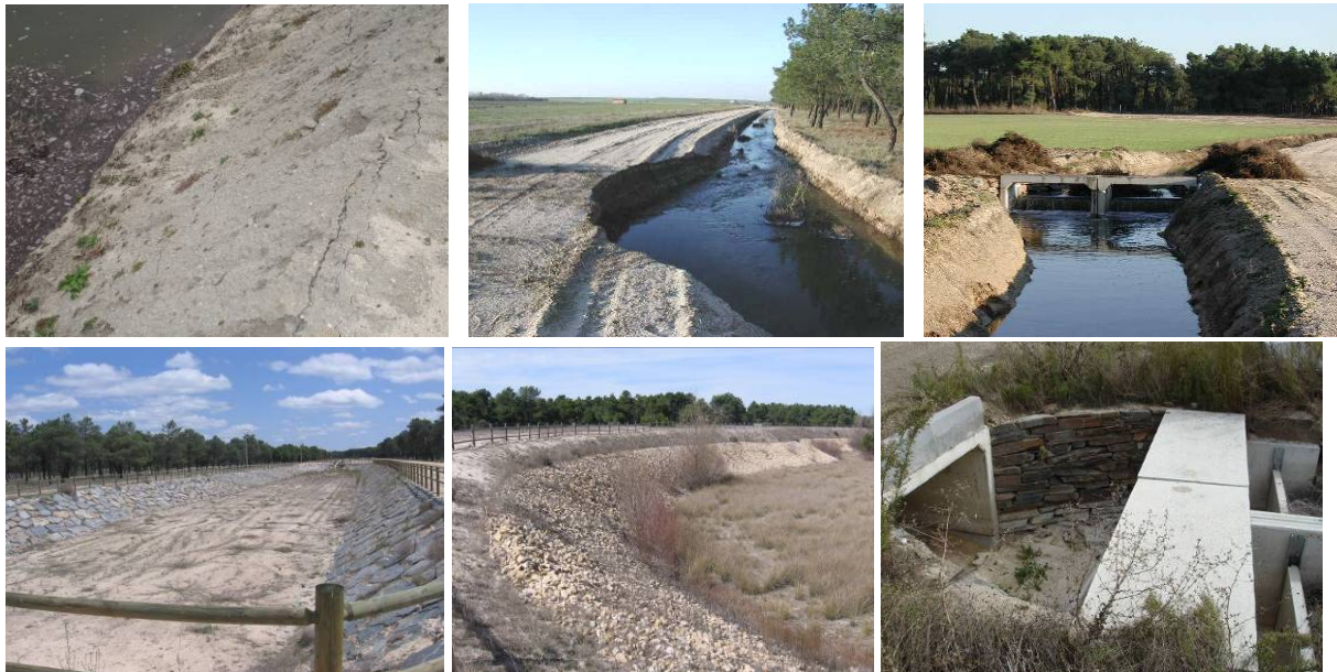
Figures 5-12 a) to f). 1/1 slope with potential slices due to desiccation processes (a, b); 2H/3V initial design (c); 3H/2V as the most common slope in the channels and ponds walls (d,e); and eventual gabions protections (f).
