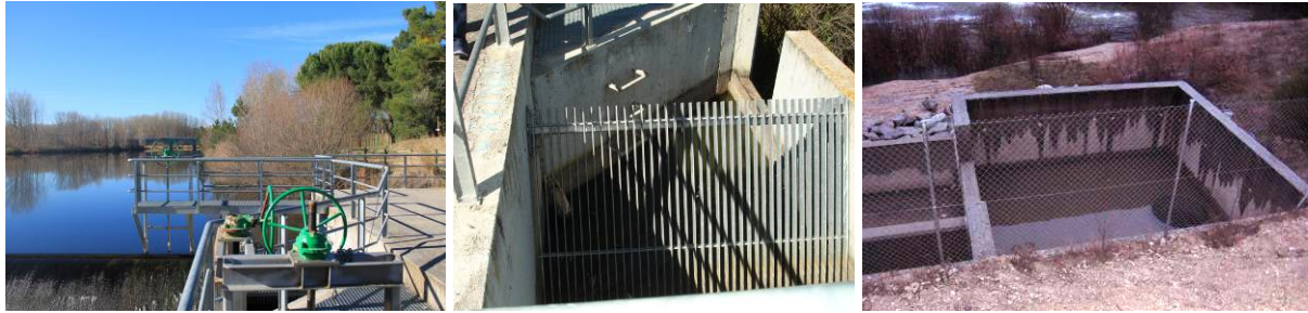
Figures 5-4 a) to c). Initial grid and filtering system in the diversion dam inlet valve in Santiuste basin and structure for stagnation in Carracillo council's catchment dam, Arenales Aquifer, Spain.
