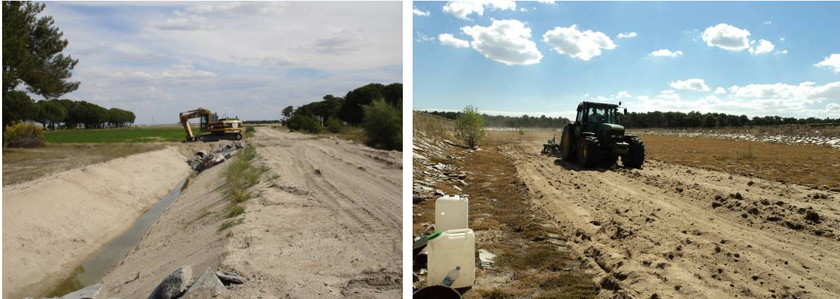
Figures 5-21 a) & b). Cleaning and maintenance operations in ponds and canal by means of excavators (sand and clogging replaced by clean sand, a) and scarification by means of tractors with adapted accessories (b).
