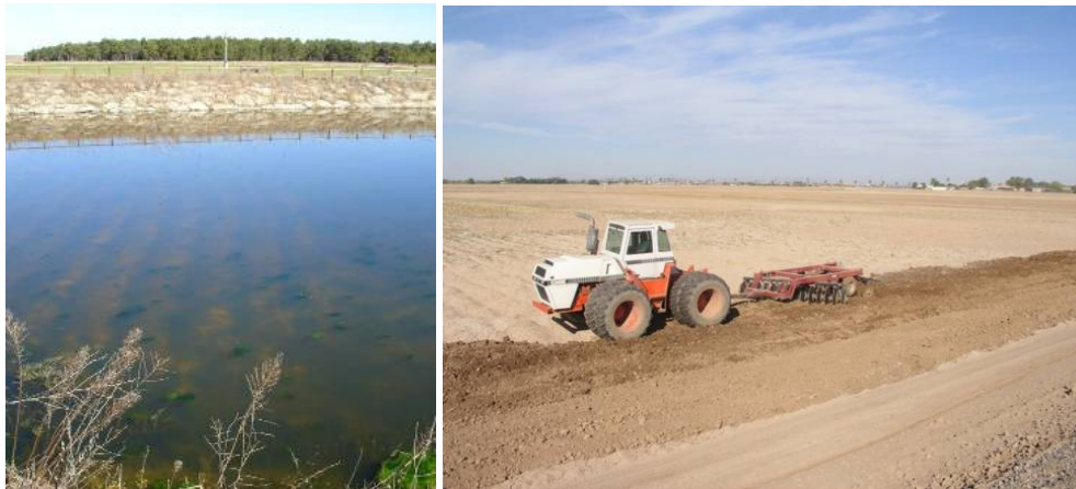
Figures 3-4 a) & b). Furrows ploughed with different width at the bottom of a decantation and infiltration pond. Headwater of the Santiuste MAR device in Spain (a) and Phoenix infiltration pond (b).
