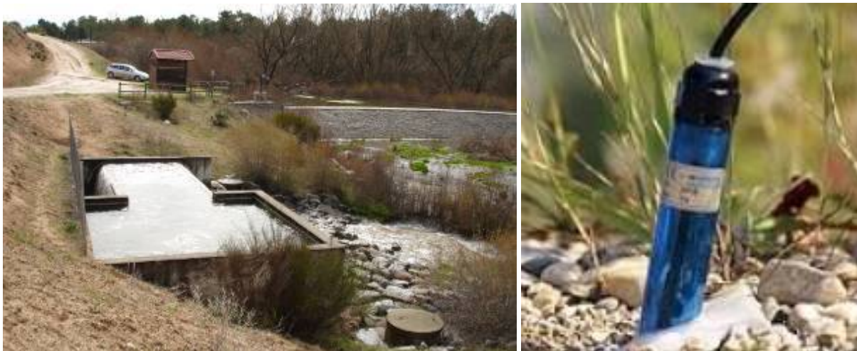
Figures 5-18 a) & b). Some examples for technical solutions already deployed in Arenales Aquifer, Spain. Stagnation system in the heading beside the river dam, modified design to avoid the shake of the water increasing the DO content (a) and systems to evaluate the evolution of gas clogging entrapped in the aquifer.
