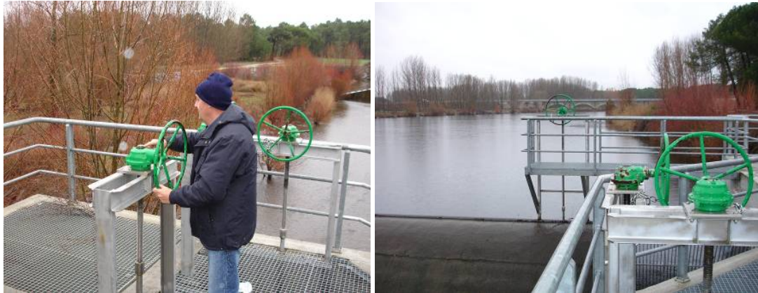
Figures 5-29 a) & b). Manual operation: Manual control of the inlet valve by farmers advised. Close on flood, storms, frost, etc.
