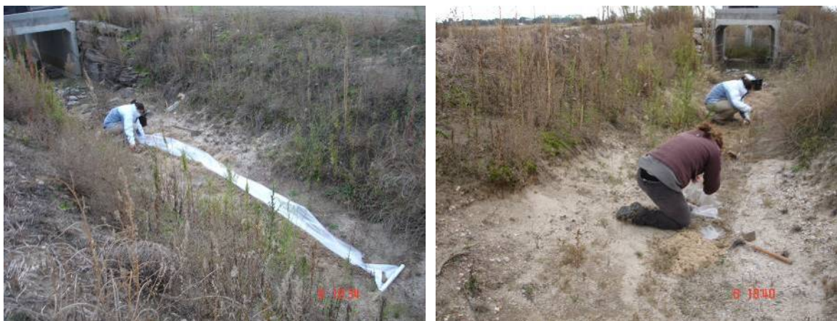
Figures 5-20 a) & b). Geofabrics installed in the bottom of the MAR canal to facilitate the cleaning of clogging processes with minor changes in the infiltration rates in Santiuste basin.
