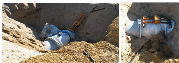
Figures 5-31 a) & b). Sand filter “in itinere” equipped with a flow meter.
