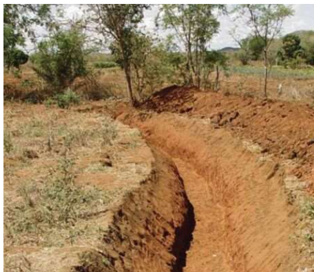
Figure 4-12: Image of a recharge trench along the contour lines to capture rainwater (Source: WCT).
