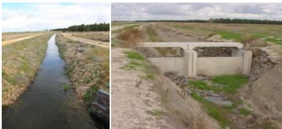
Figures 4-9 a & b: Infiltration channel in Santiuste with recharge water (a). Infiltration channel double precast stopping device in Santiuste basin (b) (Los Arenales demo-site, Spain).
