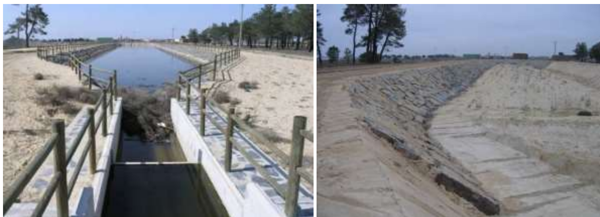
Figures 4-7: a & b. East Infiltration pond in El Carracillo District, Los Arenales demo-site (Spain).
