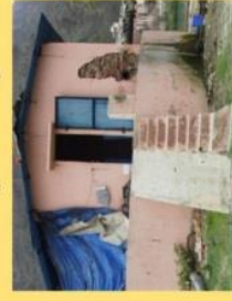
Fig. 3: RBF well in poor sanitary condition (unsealed base, cracked caisson)
