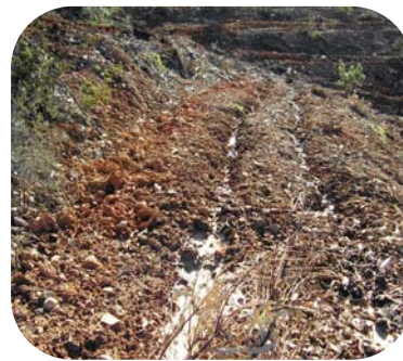
The creation of contoured furrows or ditches reduces water erosion and increases the time that the water remains on the hillside, fostering natural infiltration, aquifer recharge and the growth of plants put in place. (Photo: TRAGSATEC).
