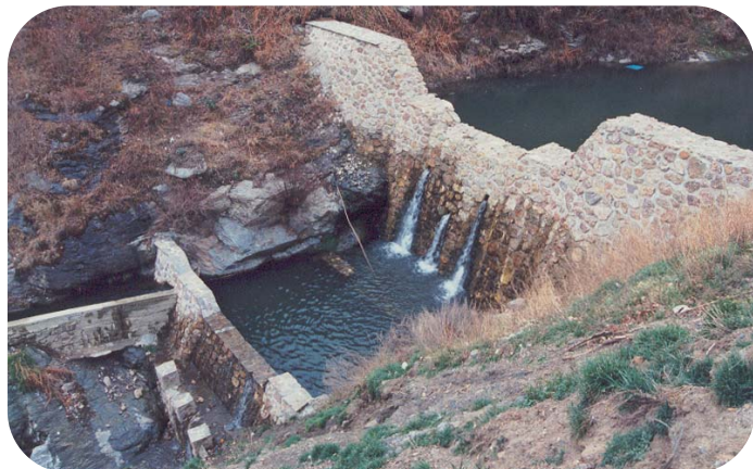
Dyke in a torrent in Sierra Nevada (Granada). It laminates the peak flow volume and increases infiltration (Photo: TRAGSATEC)
